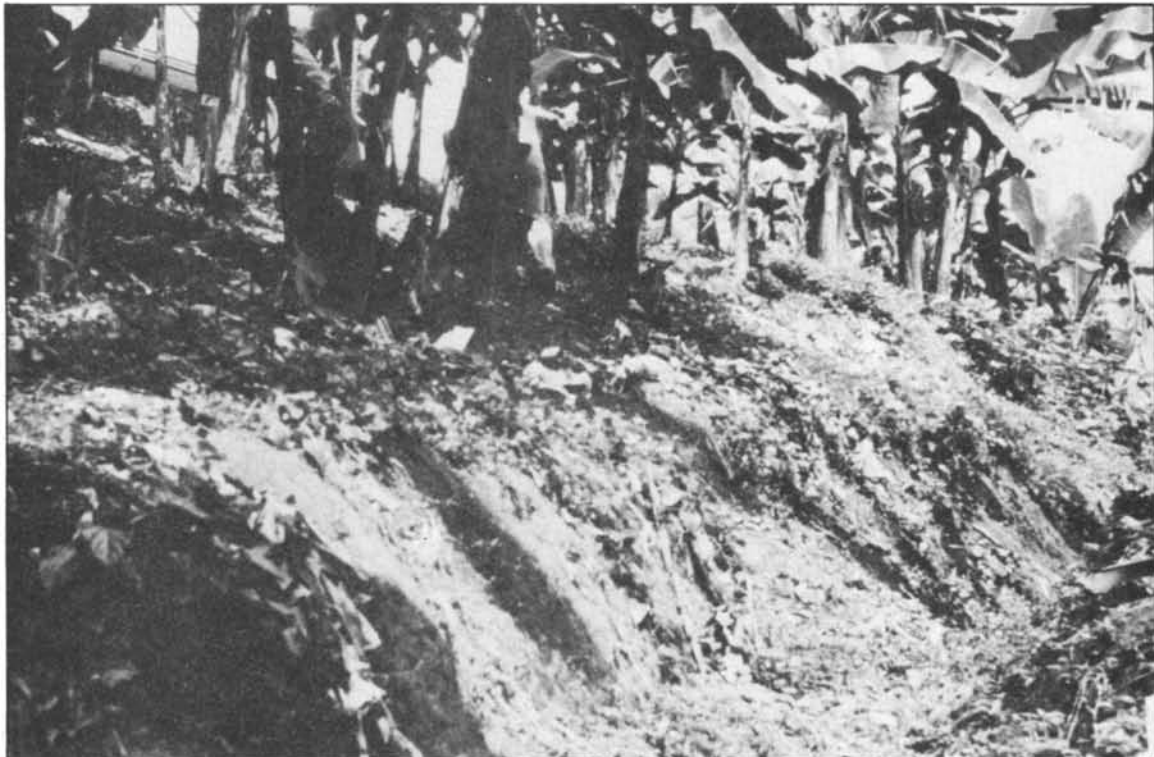
Figure 7.15 Eroded cutoff drain
